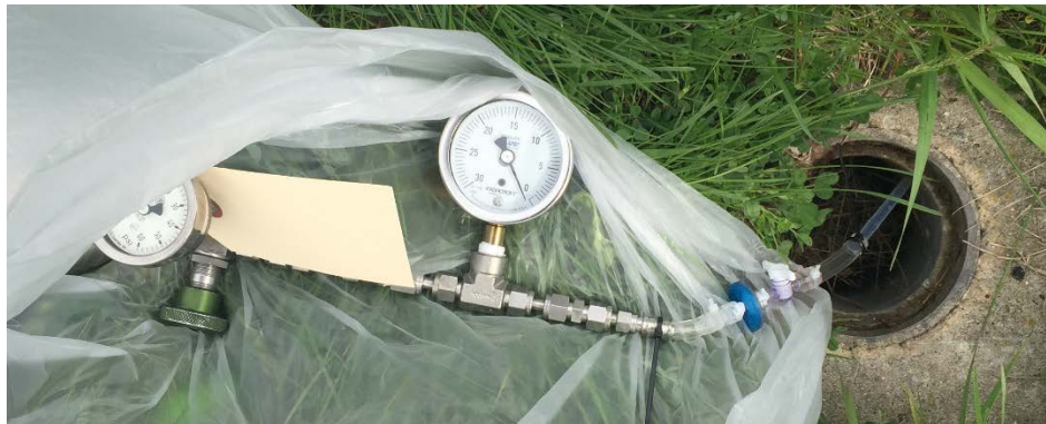
Photograph 18 – Exterior soil gas sampling point with moisture filter setup to begin shut-in leak test
