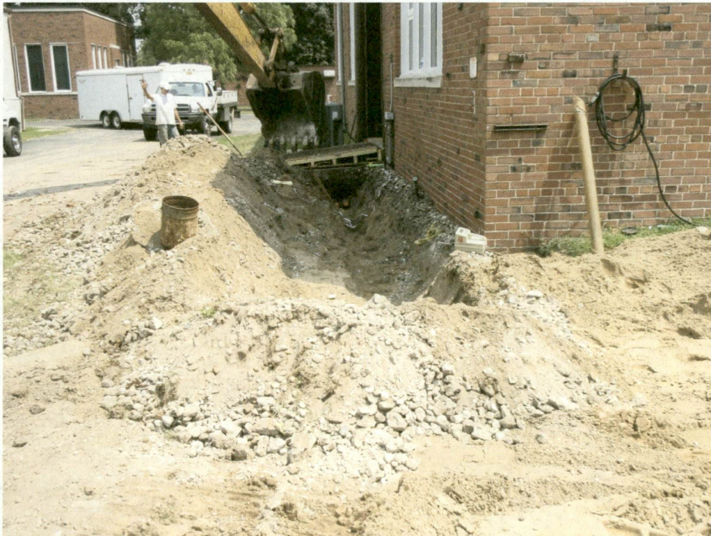
Photograph No. 8 Product piping line excavation at CMI Tech Center, Inc. facility (29 July 2008)
