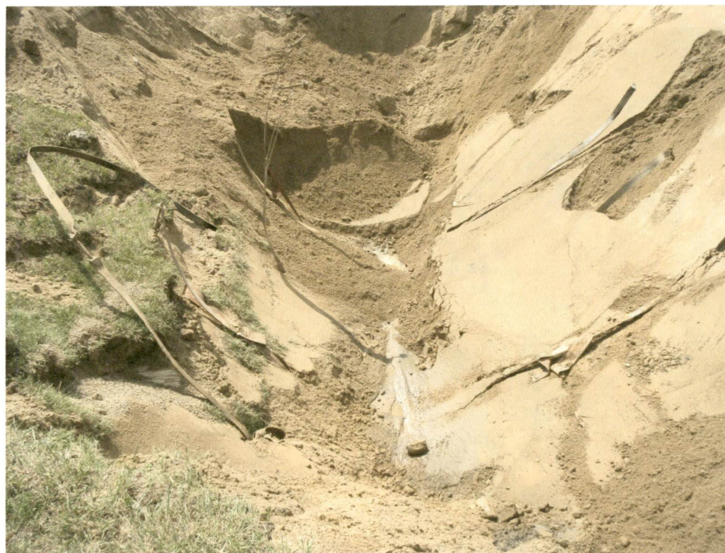
Photograph No. 4 Excavation floor beneath gasoline UST at CMI Tech Center, Inc. facility (28 July 2008)
