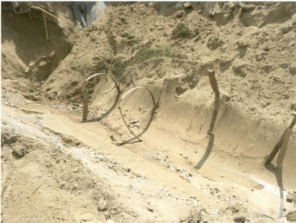
Photograph No. 2 Excavation floor beneath diesel UST at CMI Tech Center, Inc. facility (28 July 2008)
