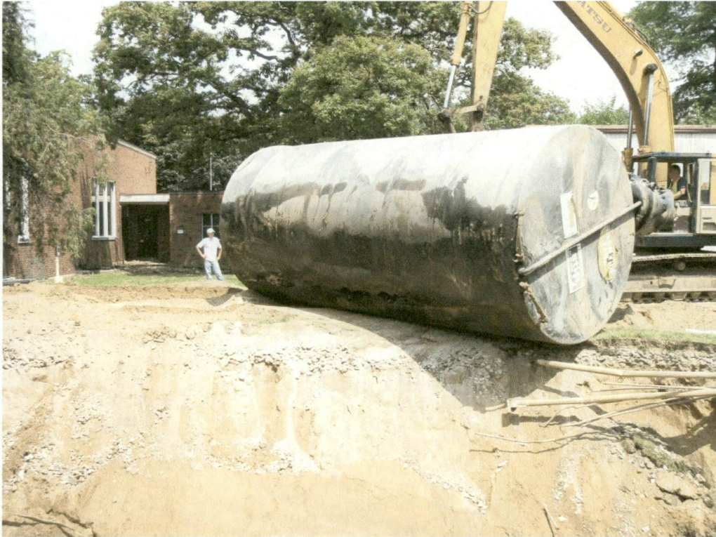
Photograph No. 1 Diesel UST removed from ground at CMI Tech Center, Inc. facility (28 July 2008)
