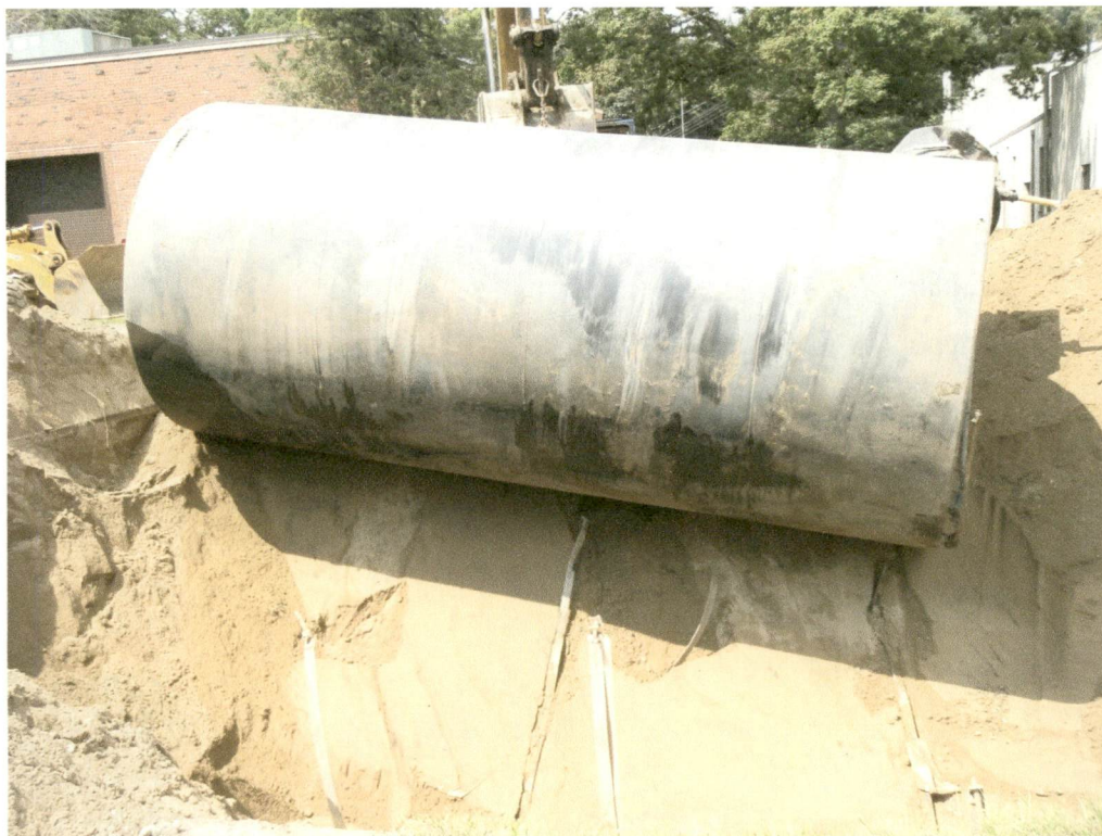
Photograph No. 3 Gasoline UST removed from ground at CMI Tech Center, Inc. facility (28 July 2008)
