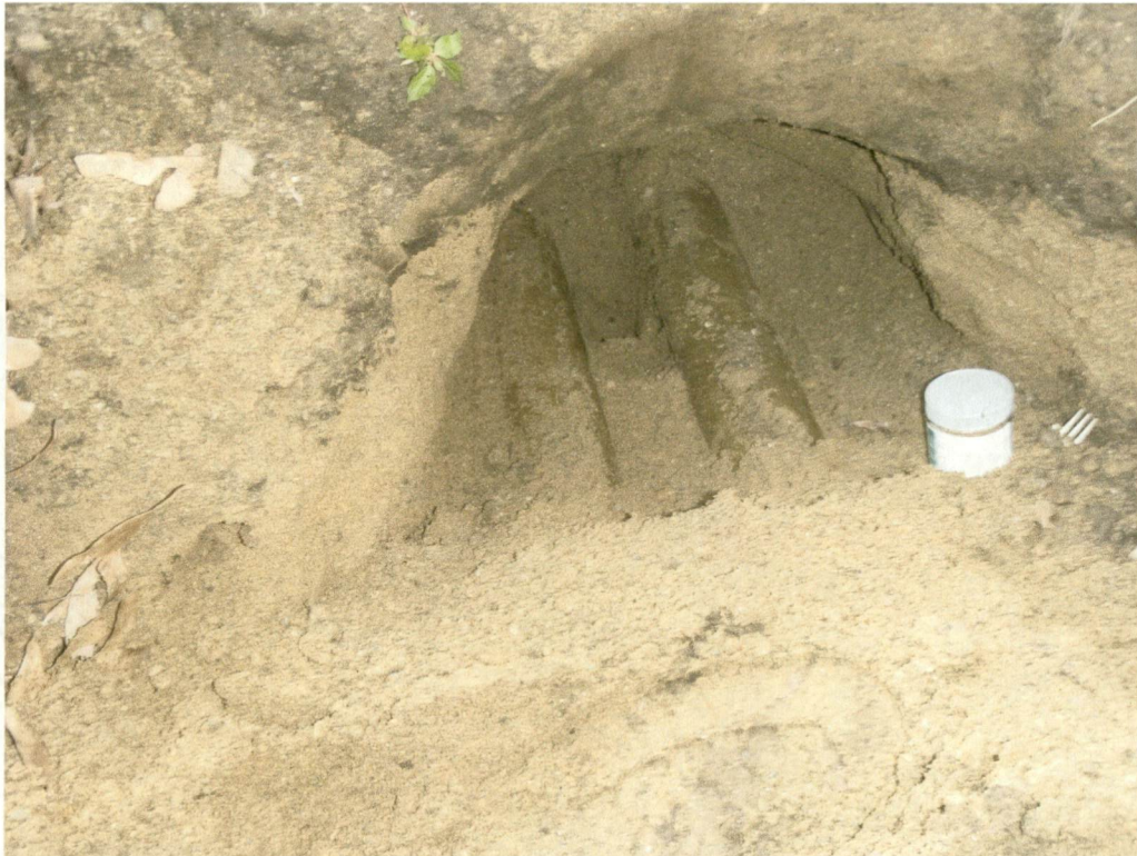
Photograph No. 7 Product piping line P-2 sample location at CMI Tech Center, Inc. facility (29 July 2008)
